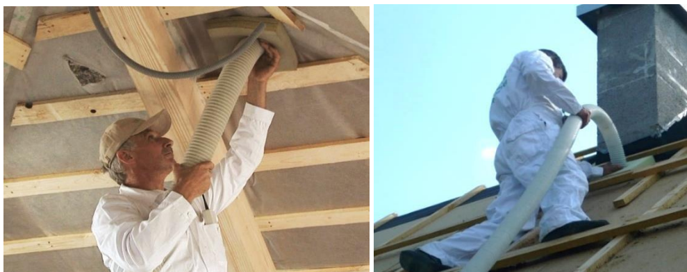
Figure 3: Cellulose insulation in a pitched roof
